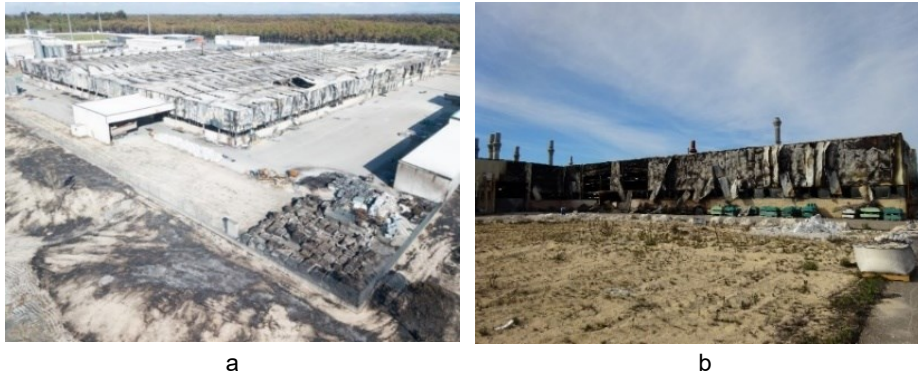
Fig.1 – Damages in external cladding in industrial buildings affected by 2017' Greatest Forest Fires
