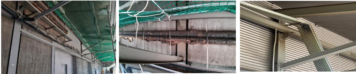
Fig. 2. Deterioration of the installations outside the building in the fire region.
