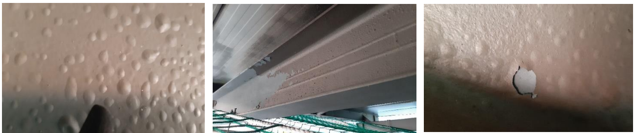
Fig. 4. Organic coating damage with bubble formation and detachments.
