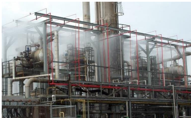
Figure 3 - Example of an automatic deluge system in a chemical plant handling ignitable liquids
