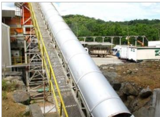
Figure 3: Catwalk to access the conveyor (Componente, 2021) [37]
