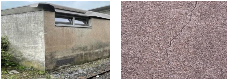
Fig. 5. Coloration of a cementitious façade of the building in the fire area. The crack width reaches 1.5 mm (right).
