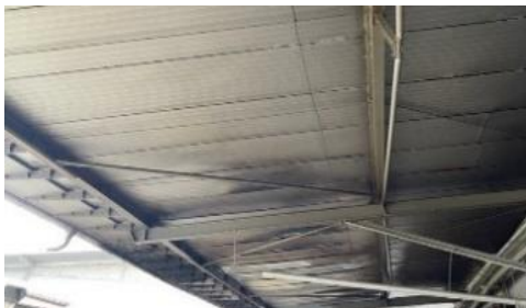
Figure 1. Fire affected zone of the industrial shed. A view of the outdoor roofing elements where the fire initiated.
