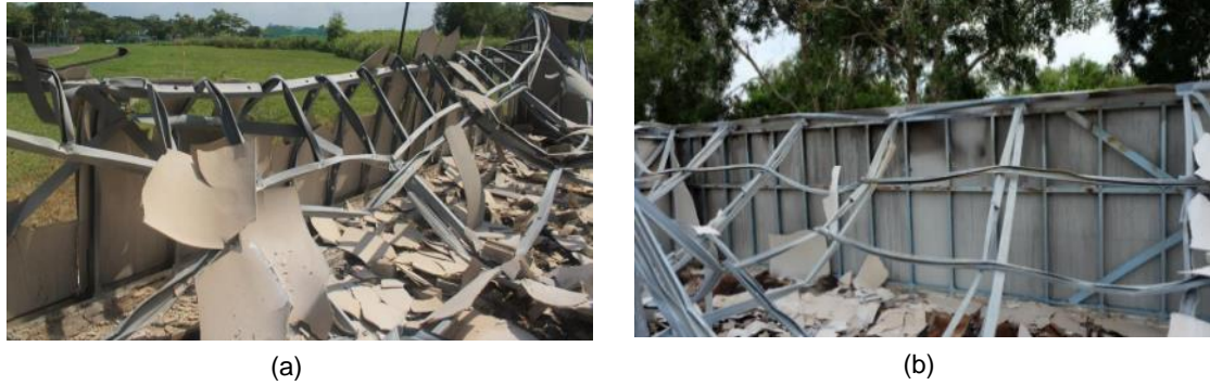
Figure 21 Influence of protection on the structure integrity. a) Northern wall, without Gypsum protection b) Southern wall with Gypsum boards [19]
